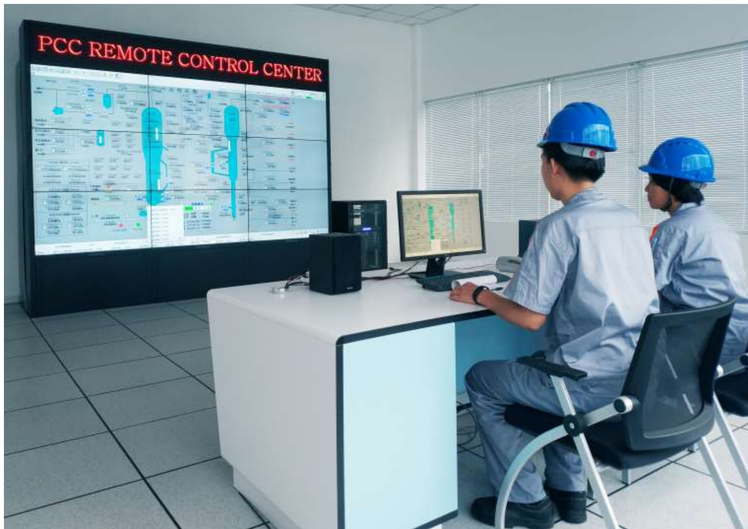
PCC Remote Control Center
