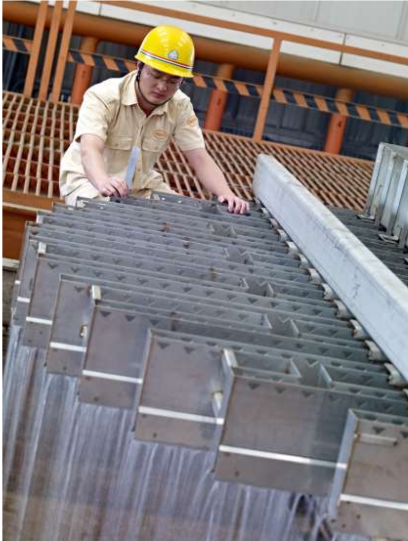
Distributor hydraulic testing
